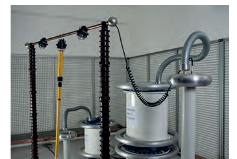
High voltage laboratory
